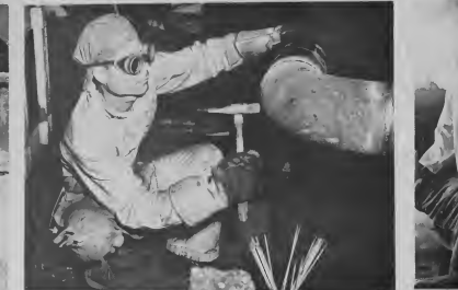
UPON completion of a welding job, excess weld is chipped off the surface. Pieces of flying weld could very easily lodge in the eye. To ward off such possible injury this employee wears protective goggles.
